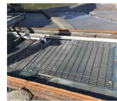
The collection grid under the slipway collects pollutants at the Royal Victoria Yacht Club.
